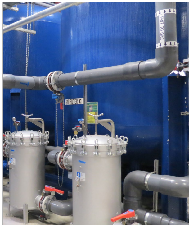
Granular Activated Carbon Tanks and Sediment Filters at SEPTS
