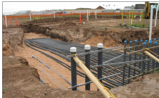
Installation of piping and manifold for a soil vapor extraction system at Pantex
