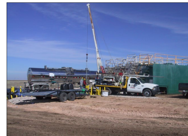
Preparing for injection of amendment to create a permeable treatment zone in perched groundwater.
