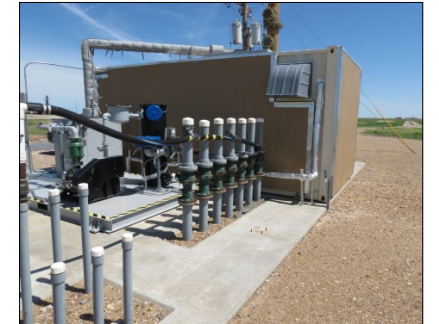
SVE System at Burning Ground
