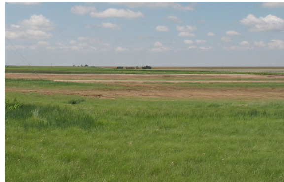
New grass takes the place of the Old Sewage Treatment Plant after demolition.
