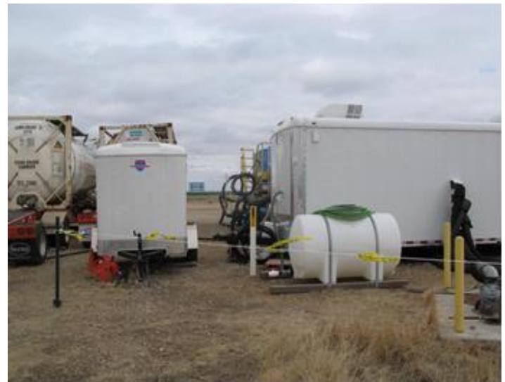
Amendment Tanks and Control Buildings at the ISBs
