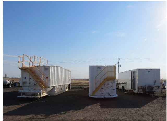
Amendment Tanks and Control Trailers at the ISBs
