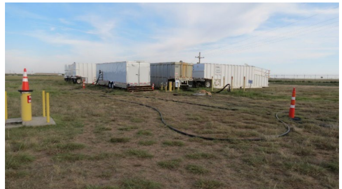
Injection Trailers at Zone 11 ISB
